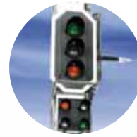
Signalling and control cables
